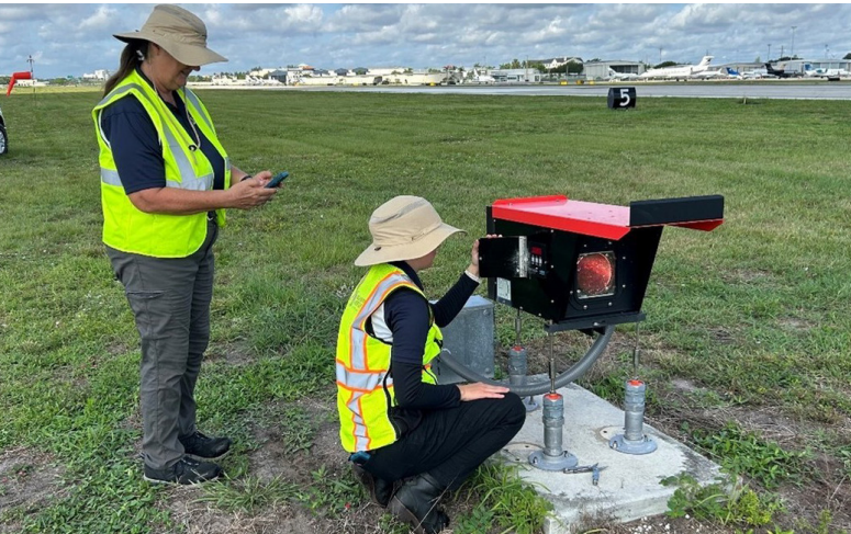
Airport Operations staff perform inspections of the PAPIs. Staff routinely inspects to make sure these vital safety tools are correctly calibrated and are easily visible to pilots on approach.
