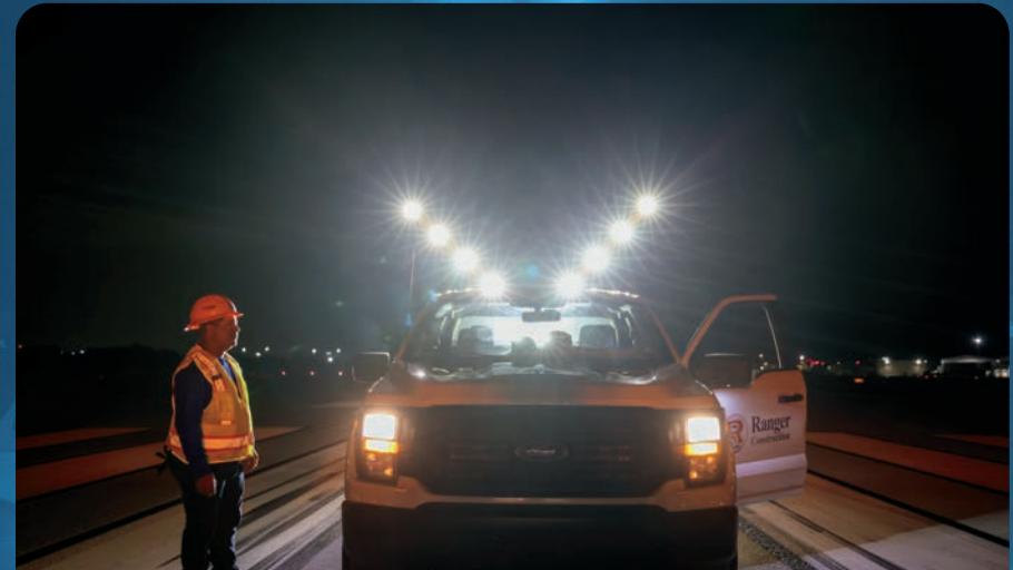
Boca Raton Airport utilized Halibrite X illuminated closure markers for the first time in early September 2025, enhancing visibility and safety during runway construction and rehabilitation.
