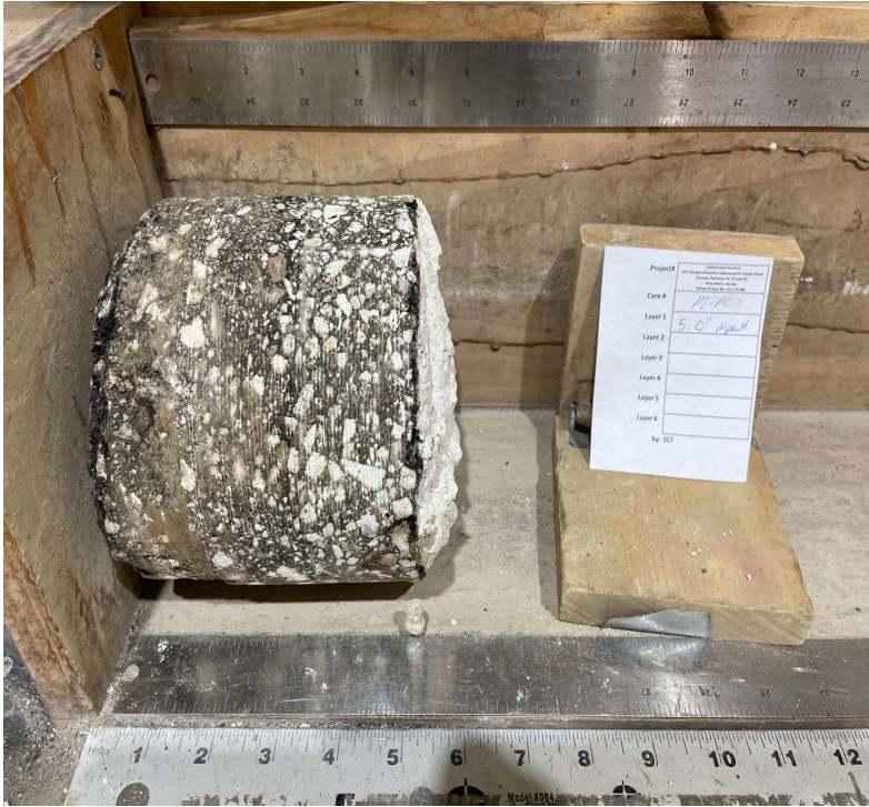
Core ID PC-P2C1 Core Date 11/12/2025 Latitude 26.384535 Longitude -80.10227 Pavement Layer 1 5 Total Core Length (in.) 5 Base Material Thickness (in.) 1 LR 12 Stabilized Subgrade? N/A Comments STABILIZED SUBGRADE NOT APPARENT. BASE COURSE UNDERLAIN BY LIGHT BROWN SAND.
