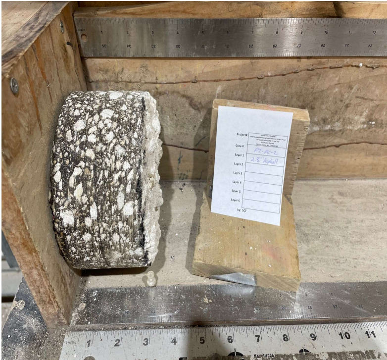
Core ID PC-P2C2 Core Date 11/12/2025 Latitude 26.384632 Longitude -80.102364 Pavement Layer 1 2.8 Total Core Length (in.) 2.8 Base Material Thickness (in.) 1 LR 11 Stabilized Subgrade? N/A Comments STABILIZED SUBGRADE NOT APPARENT. BASE COURSE UNDERLAIN BY BROWN SAND.
